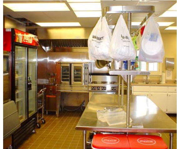
Large Commercial Kitchen With Ice Machine & Large Refrigerator
